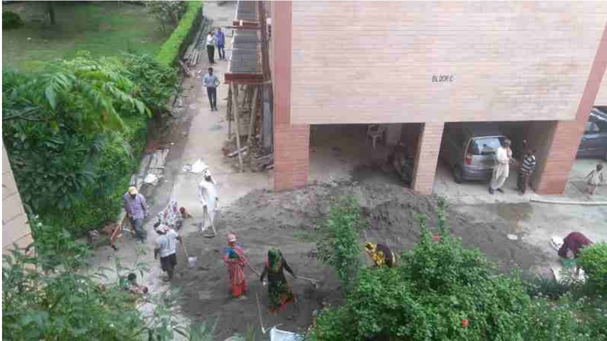
Deadly dust and noise pollution is caused by illegal construction in a cooperative group housing society of Dwarka, New Delhi
